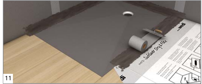
11 Seal the joins and timber beam transitions with the wedi Fundo sealing set. Recommendation: Seal the complete timber floor area with wedi Dry & Flex.
